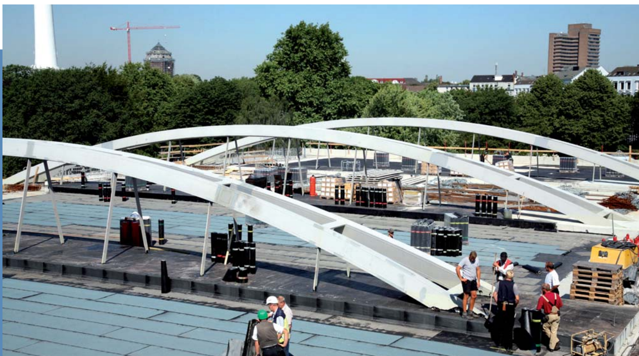
The roof of the CCH's multifunctional exhibition hall was completed in 2006. The largest rooftop garden in Europe is being created here in 2007.
